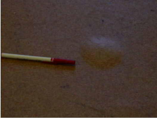
FIGURE 8, Disbonding from Moisture Vapor Transmission
