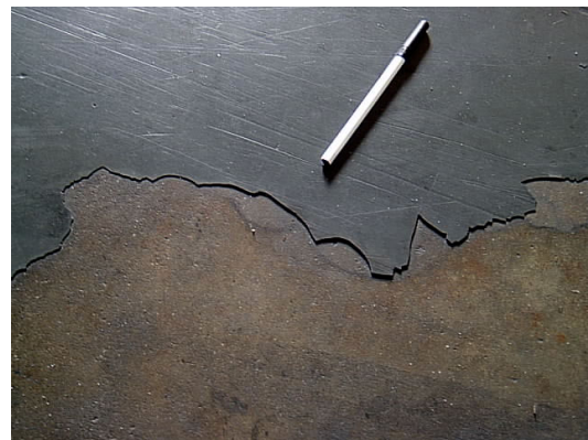
FIGURE 4, Bond Failure at Substrate.
